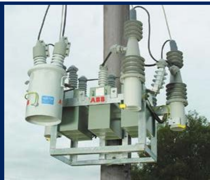
3 pole mounted HV capacitors
