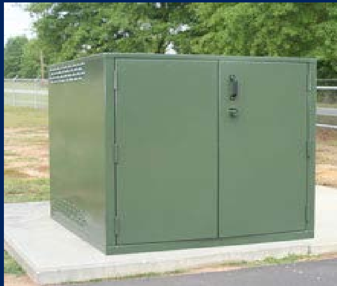
4 ground mounted HV capacitors
