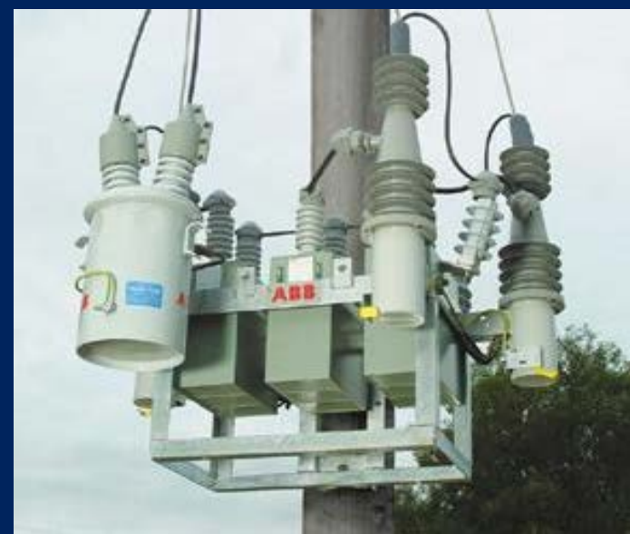
4 pole mounted HV capacitors
