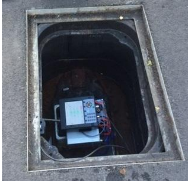
Figure 3: Lynx installation, Denton East
