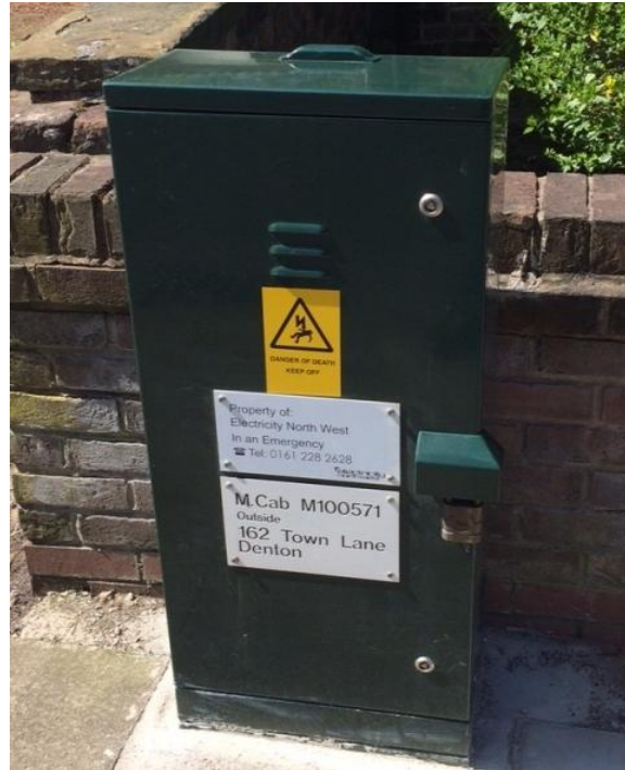
Figure 7: EPM installation, Denton East.
