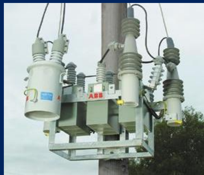
4 pole mounted HV capacitors
