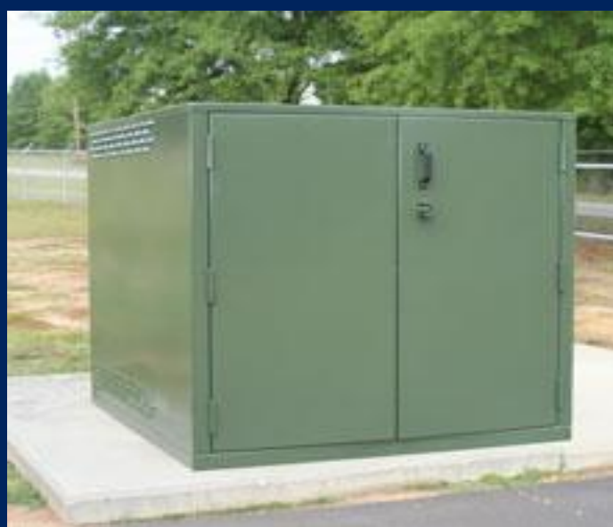
4 ground mounted HV capacitors
