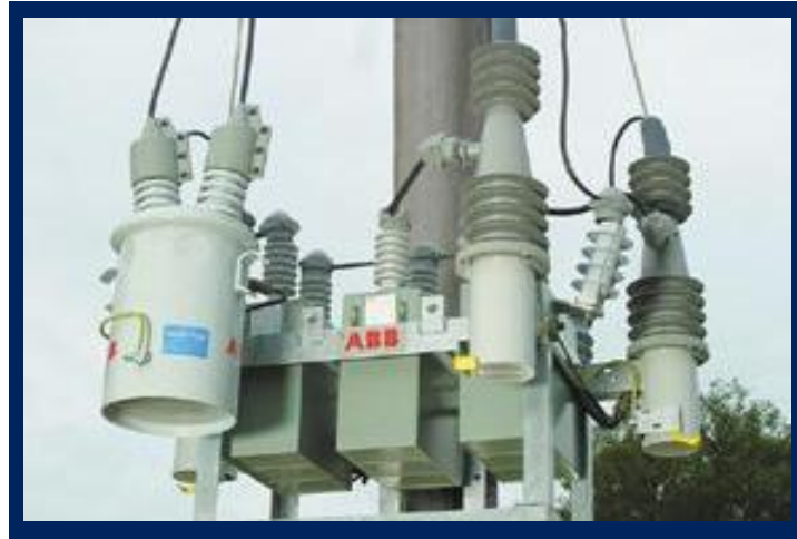
4 pole mounted HV capacitors
