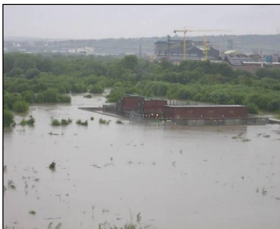
Photograph 11 - An electricity substation protected by flood barriers in the 2007 floods in the North East of England
