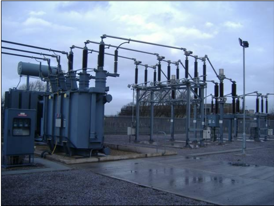
Photograph 18 - 132kV Grid Substation showing main power conductors at high level but control circuits located in cubicles at lower level
