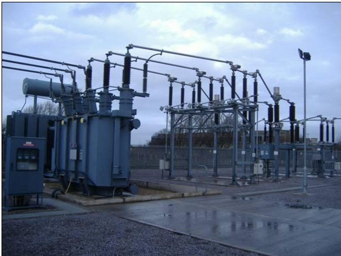
Photograph 8 - 132kV Grid Substation showing main power conductors at high level but control circuits located in cubicles at lower level
