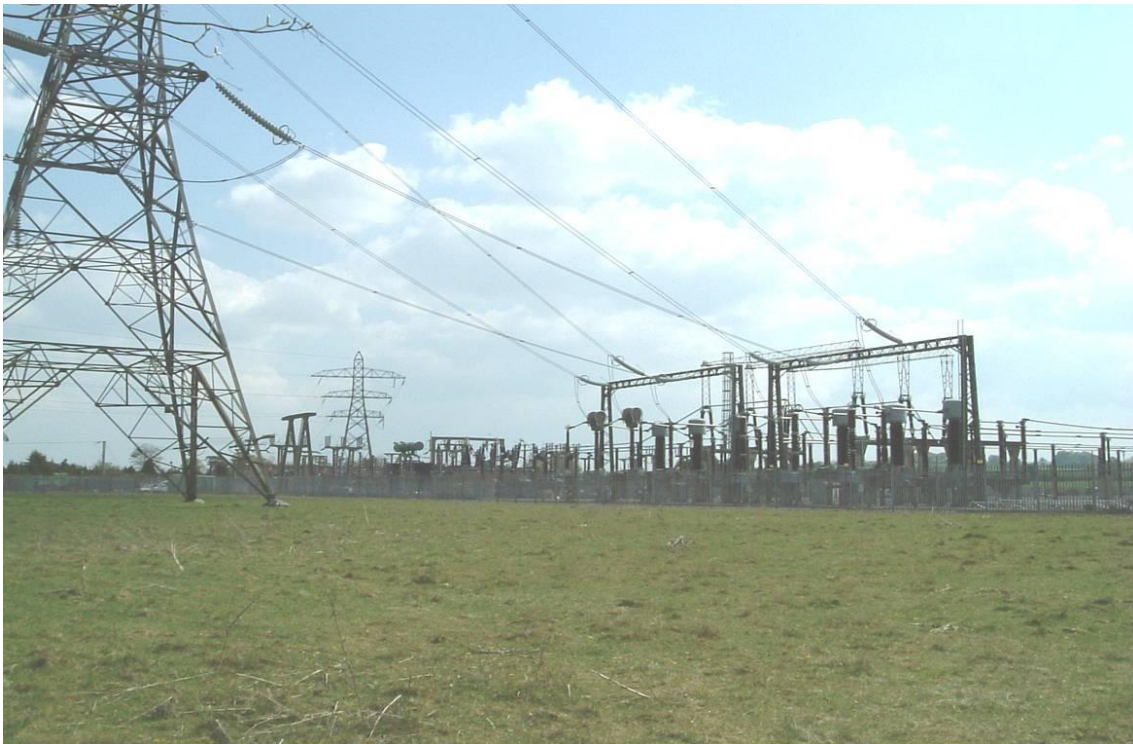
Photograph 14 - 400kV Grid Substation showing 400kV terminal tower (pylon)
