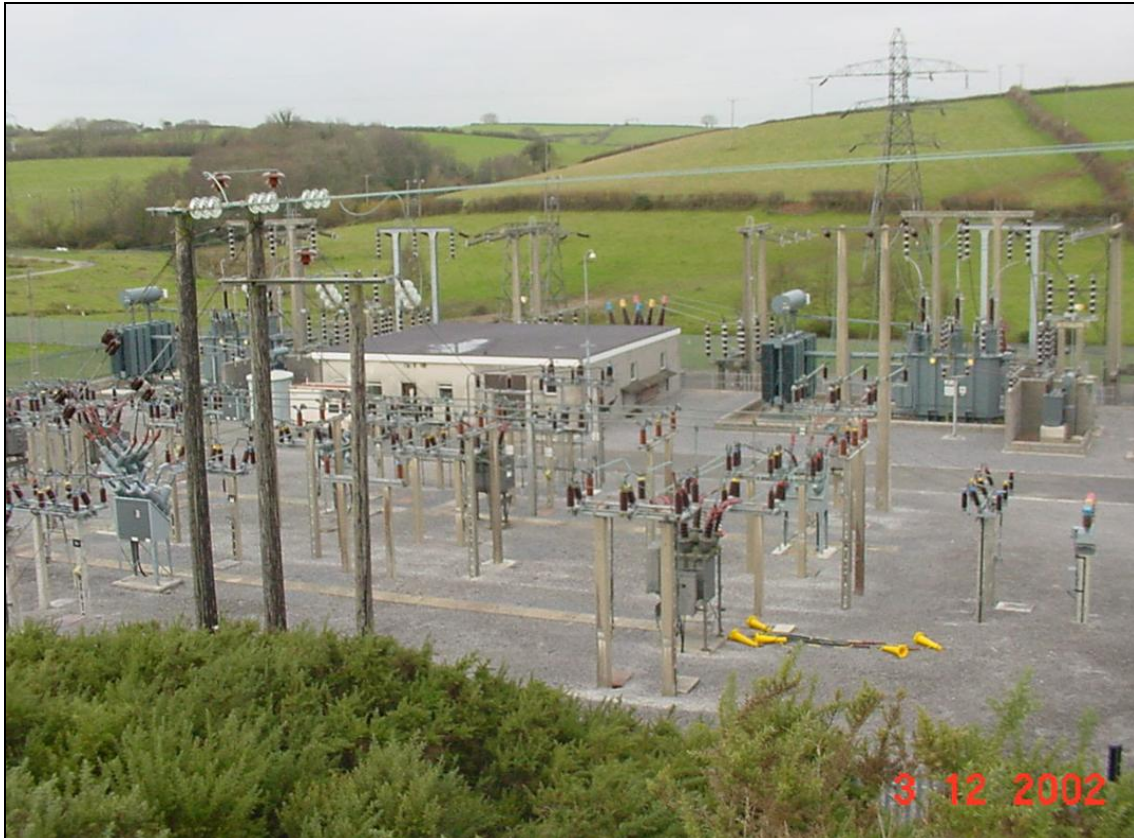
Photograph 15 - 132kV Grid Substation showing 132kV terminal tower (pylon) and start of 33kV wood pole overhead line
