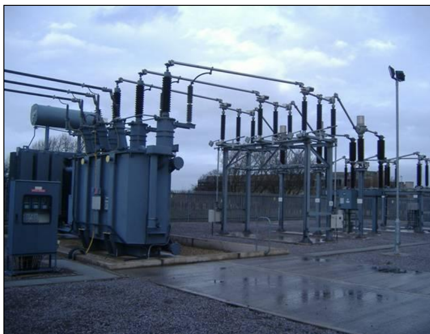
Photograph 3 - 132kV Grid Transformer and circuit breakers in service in the UK
