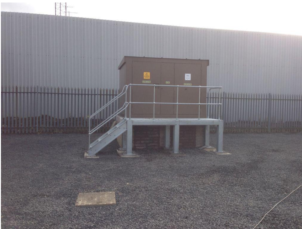
Control equipment protected on a raised plinth with step access. (Courtesy NIE)
