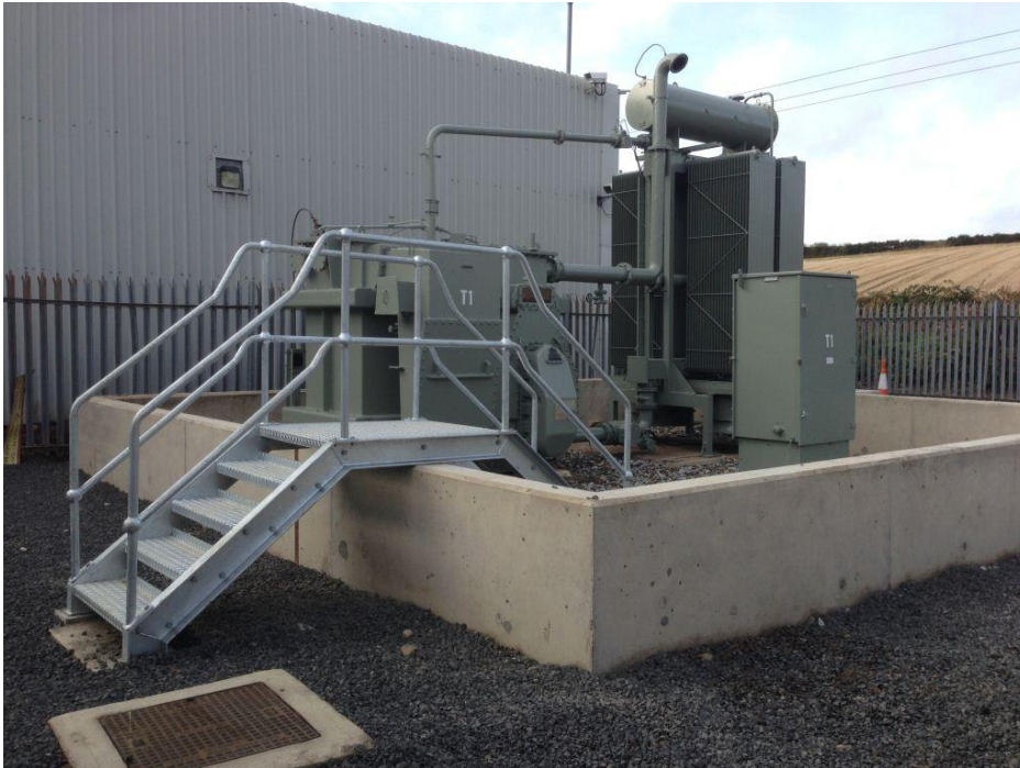
High voltage transformer and associated control equipment protected by a bund wall with step access. (Courtesy NIE)
