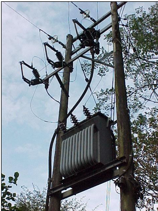
Photograph 7 - A pole mounted distribution transformer with external cooling tubes
