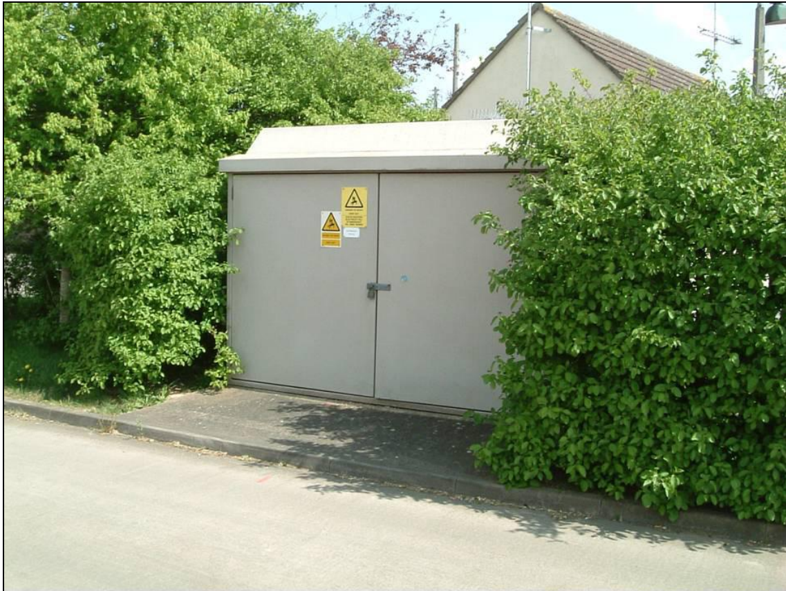
Photograph 10 - Distribution Substation with equipment operating at 11kV and 400/230 volts
