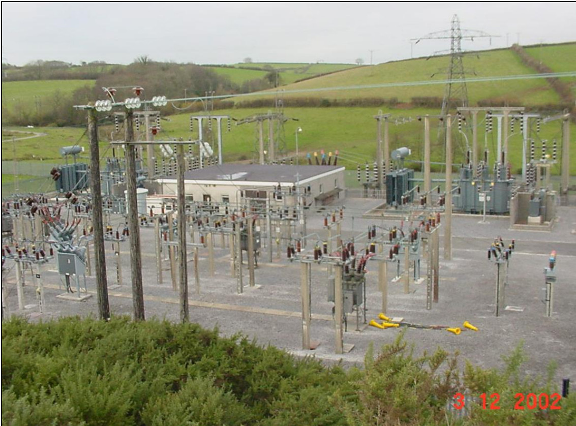
Photograph 15 - 132kV Grid Substation showing 132kV terminal tower (pylon) and start of 33kV wood pole overhead line
