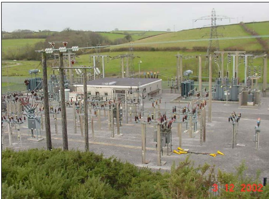
Photograph 9 - 132kV Grid Substation showing 132kV terminal tower (pylon) and start of 33kV wood pole overhead line.
