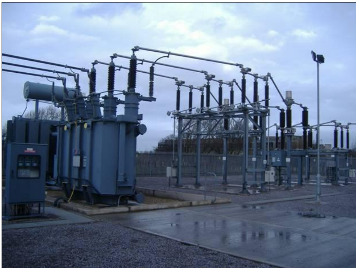
Photograph 8 - 132kV Grid Substation showing main power conductors at high level but control circuits located in cubicles at lower level
