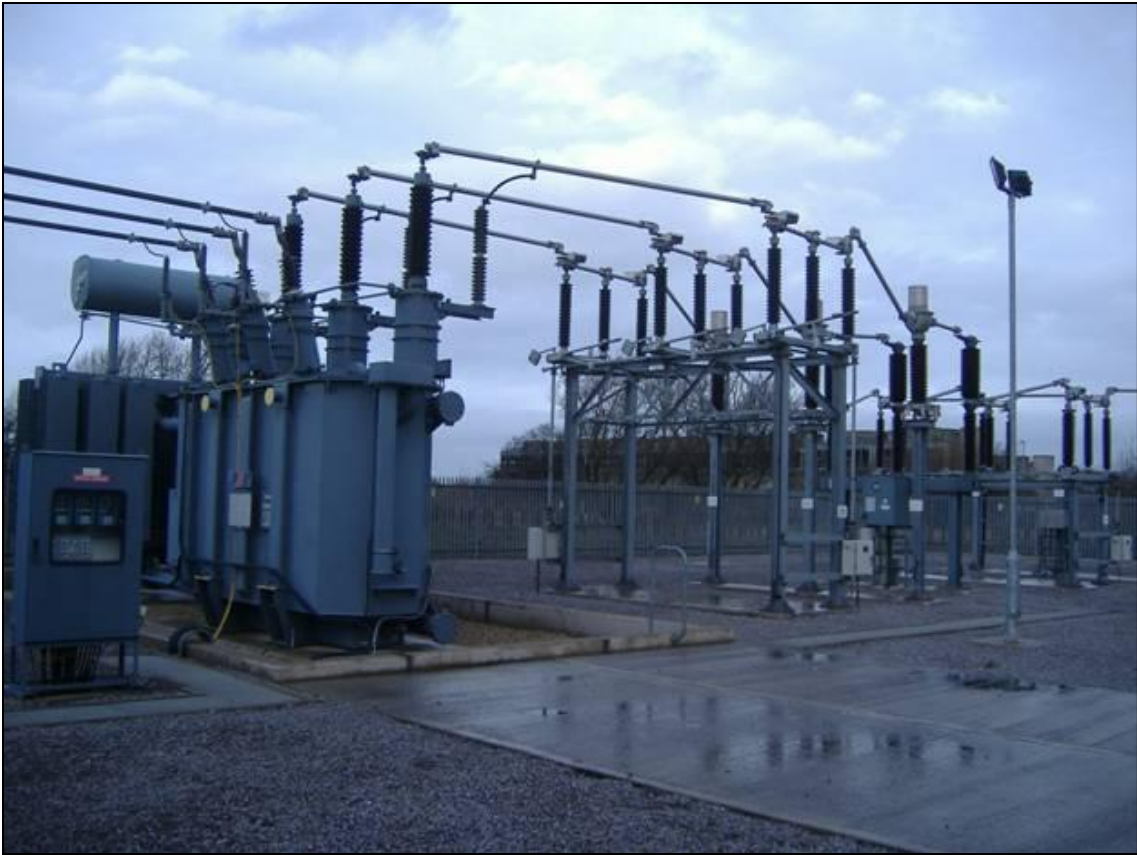
Photograph 18 - 132kV Grid Substation showing main power conductors at high level but control circuits located in cubicles at lower level
