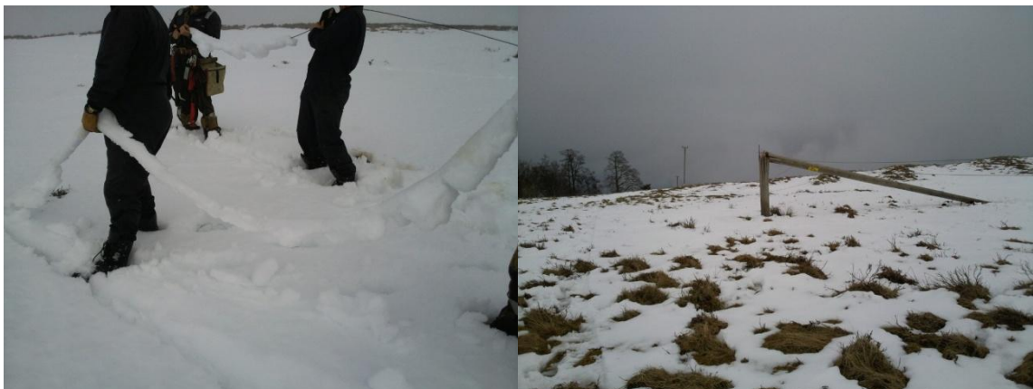
Photograph 4 - The effect of icing on an 11,000 volt rural overhead line in North West England in January 2010
