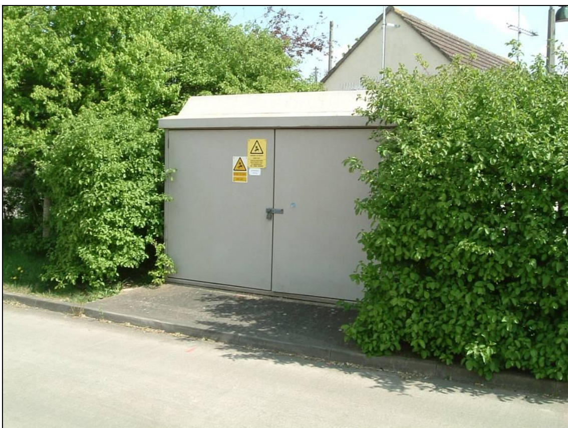
Photograph 17 - Distribution Substation with equipment operating at 11kV and 400/230 volts
