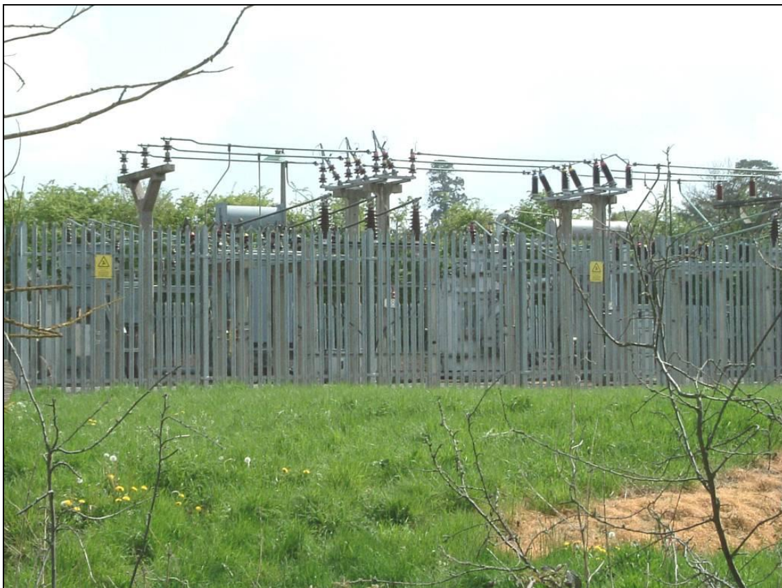
Photograph 16 - Primary Substation showing equipment operating at 33kV and 11k
